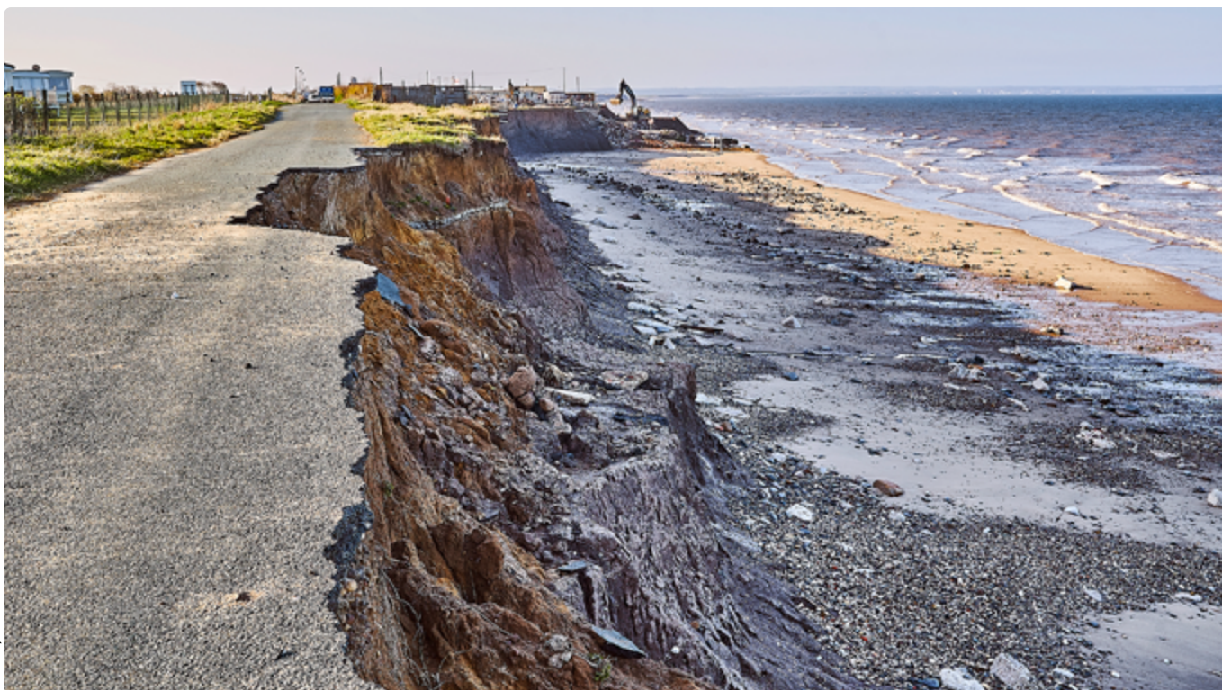
Coastal erosion at Skipsea on the East Yorkshire coast
